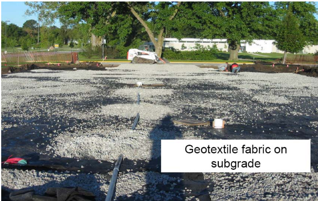
Figure 2: Placement of geotextile and aggregate subbase on subgrade (Lot 121, Iowa State University, 2007)
