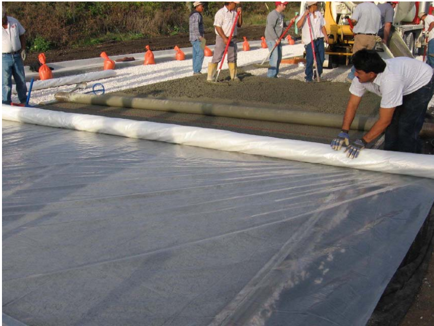
Figure 11: Covering fresh pervious concrete with plastic for 7 day moist curing period (ISU Lot 122, 2006)
