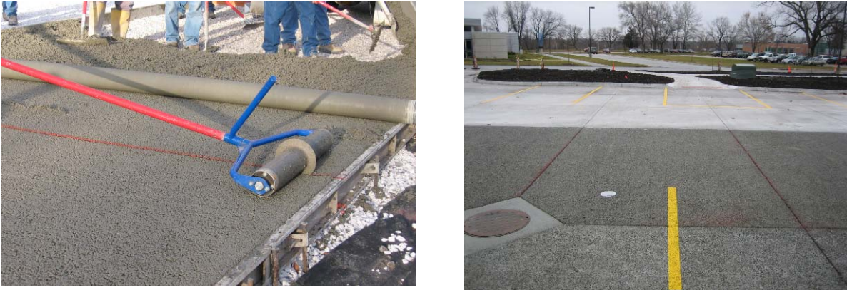
Figure 2: Jointing for pervious concrete pavement (a) Installation of joint during pervious placement (b) Joint pattern and block-outs in pervious concrete (Lot 122, Iowa State University, 2006)
