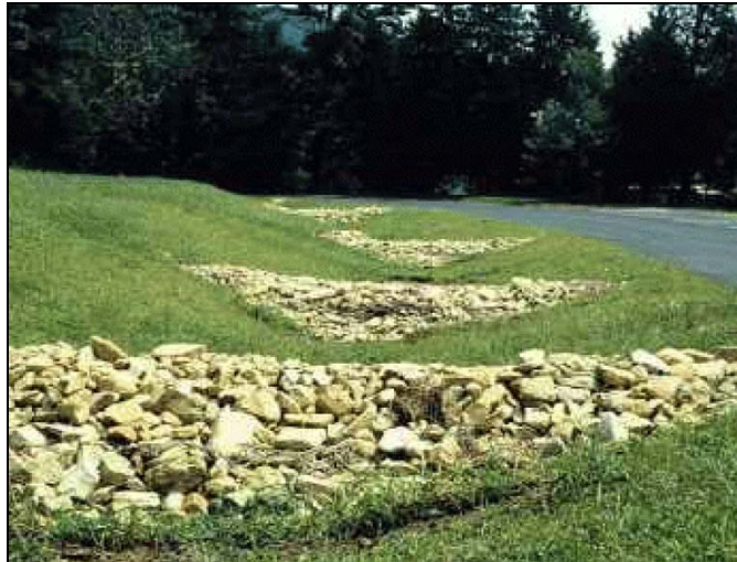
Figure 2: Grass swale with check dams (berms)
