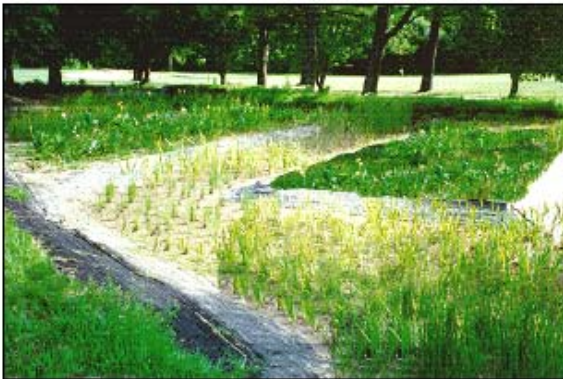
Newly Constructed Shallow Wetland
