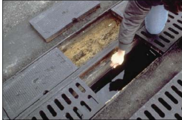
Figure 6: Perimeter sand filter
