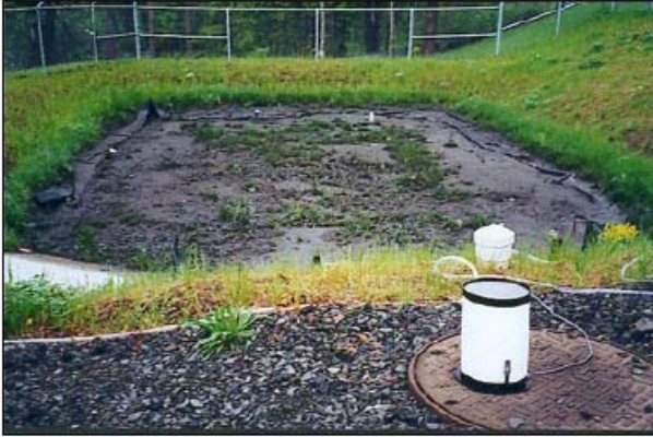
Figure 5: Surface sand filter
