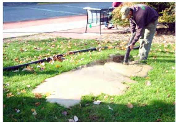
Drilling fluid at ground surface resulting from frac-out
