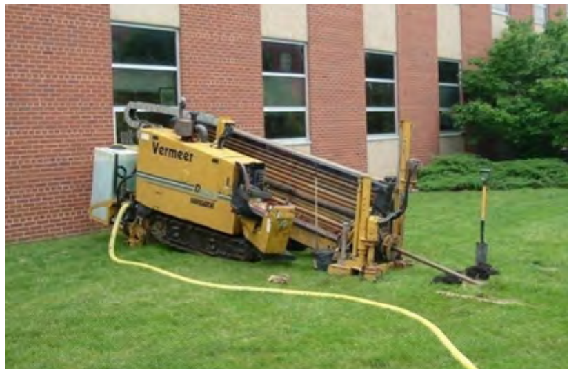
Horizontal directional drilling machine used for a trenchless construction project in Ames, Iowa
