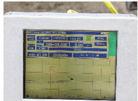
Sample screen from stringless paving control computer
