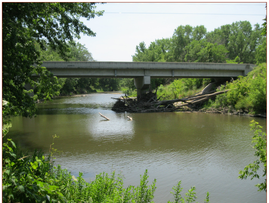
Debris accumulation at a bridge pier on the Skunk River in Ames, Iowa
