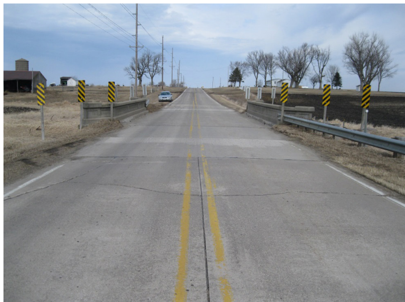
Rural Iowa farm-to-market road that has concrete bridge deck in fair condition with numerous pits and popouts, spalled and crumbling fascia, and steel girders in satisfactory condition (Image: Bridge Engineering Center)
