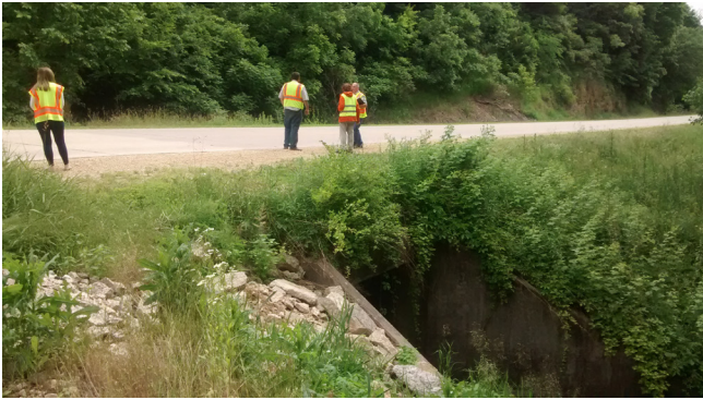
Field review near an unprotected culvert on a secondary roadway on a previous RSA conducted in Iowa
